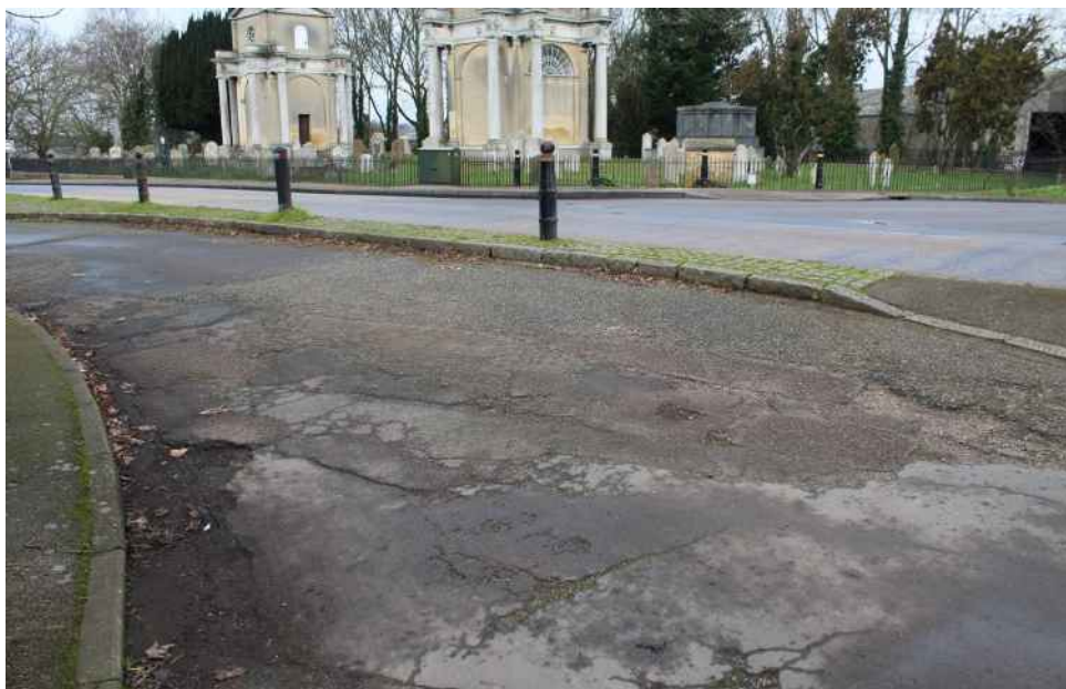
Figure 162 Poor surface treatments opposite Mistley Towers
